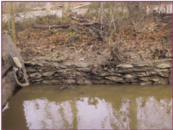
Remnants of the Skirting Canal at Violette's Lock. Photo by Norman Metzger
