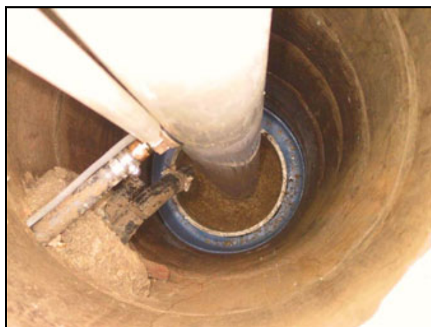
The top of the gravel pack (surrounding the white PVC tube) is 13 feet below ground level; the well itself is much deeper, down 11 feet more.
