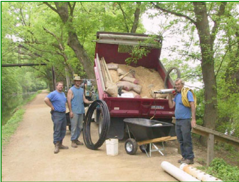
At the ferry landing. Well digging operations call for lots of equipment and materials. All hauled over on the ferry.
