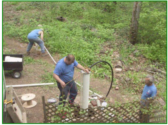
The Easterday crew measuring and testing the new installation behind the Caretaker's quarters.
