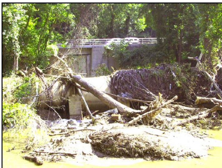
The recent heavy rains left destruction along the canal. This picture shows how an overflowing Little Falls Creek, normally carried under the canal, has washed away an embankment into the canal. Near Lock 5.
