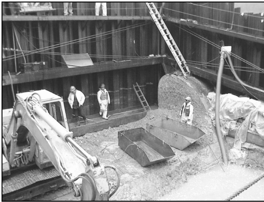
Inside the cofferdam. Debris from the dam-cut is scraped up by a backhoe into buckets for removal. Water leaking into the cofferdam is pumped out through the hose on the right. River level is about ten feet above the buckets.
