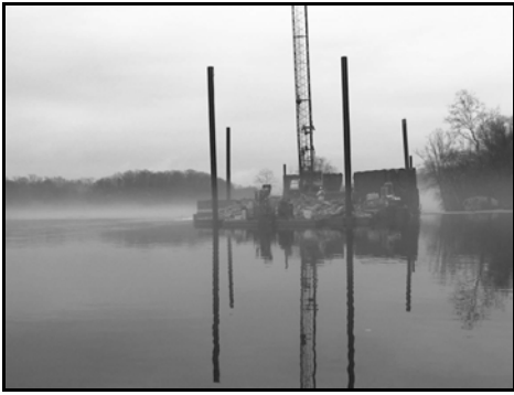
Cofferdam and crane about a mile below Sycamore Island near the Virginia shore.
